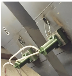
Single Impact Air Knockers were installed on two hoppers at Ebberts Field Seeds. Product now flows freely out of the hoppers and into the 50-pound bags.
